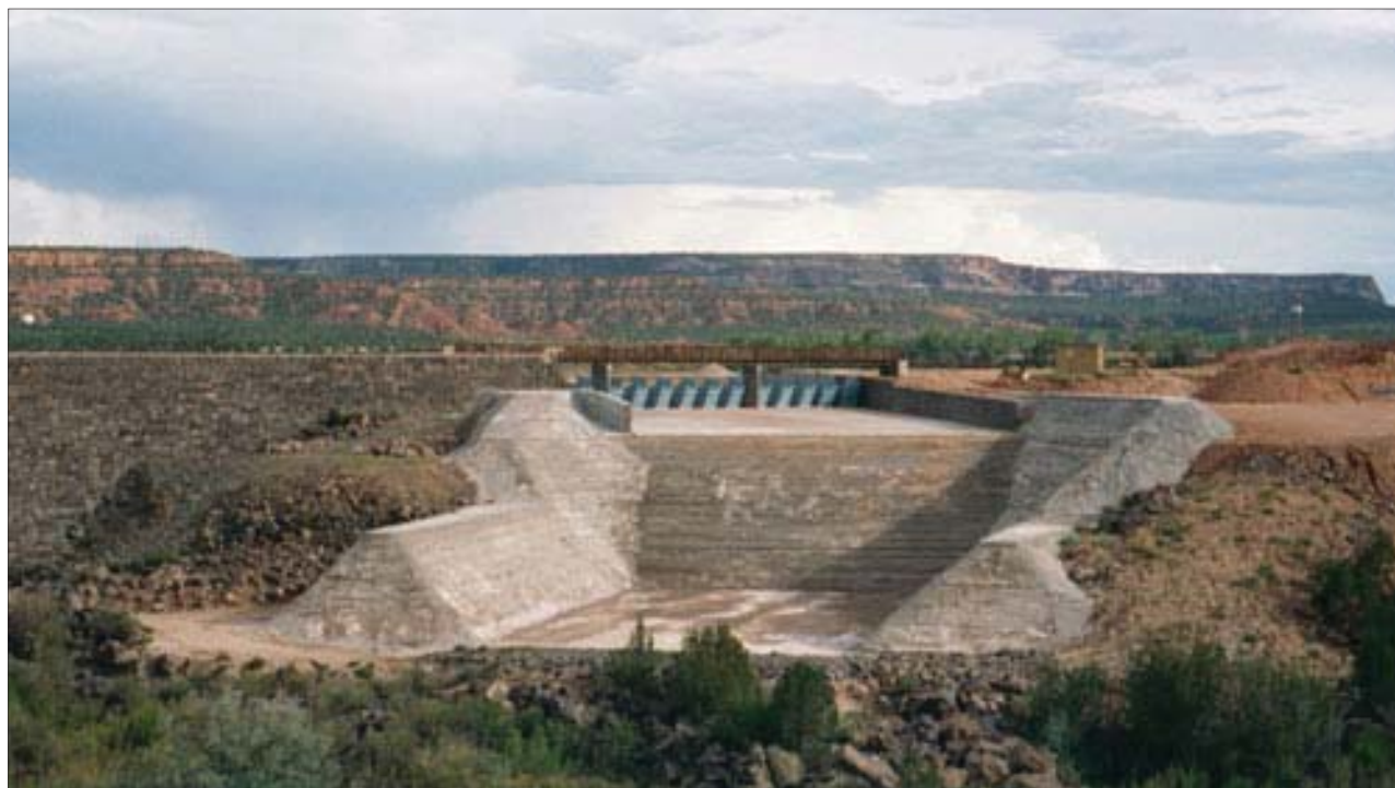
The Black Rock Dam in the Black Rock Irrigation Project. Photo source: Gannett Fleming (2002); reproduced with permission of Gannett Fleming, Inc.
